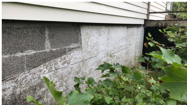
Lecamur mangler murpuss.
